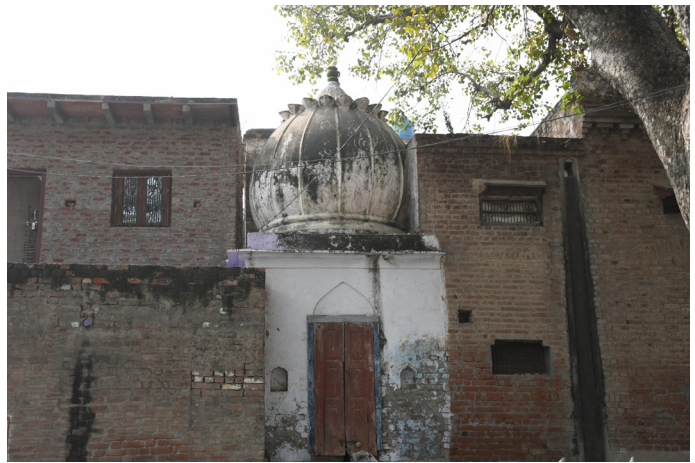
Figure 3 : Shiva and Hanuman Temple, Kasganj Tehsil Source: Primary survey by AH Division, INTACH Team
